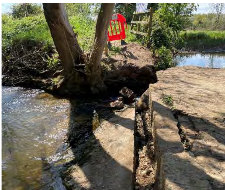
Failed spillway at Ufford with dry riverbed beyond (top right)
