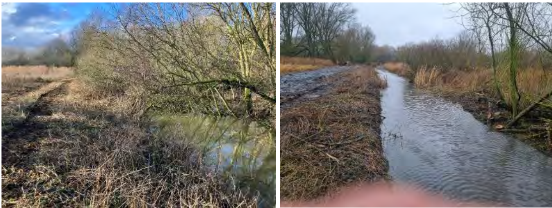
1750m of desilt and vegetation removal completed. Before (left) and after (right) shown above.
