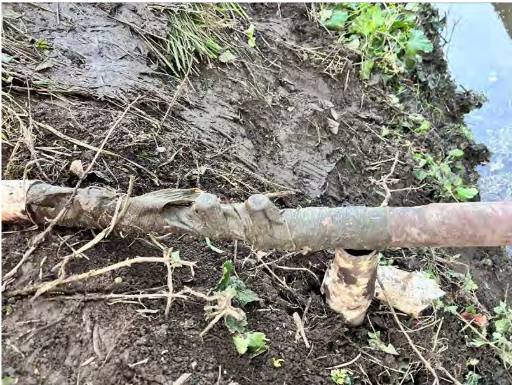
A close up of the repair – the duct has been cut and the plastic pipe repaired and then wrapped in tape. The section of removed duct has been shoved under the remaining duct to support it. It is not known if this is just a temporary repair, but it seems sub-standard for the location of the pipe considering its susceptibility to further damage
