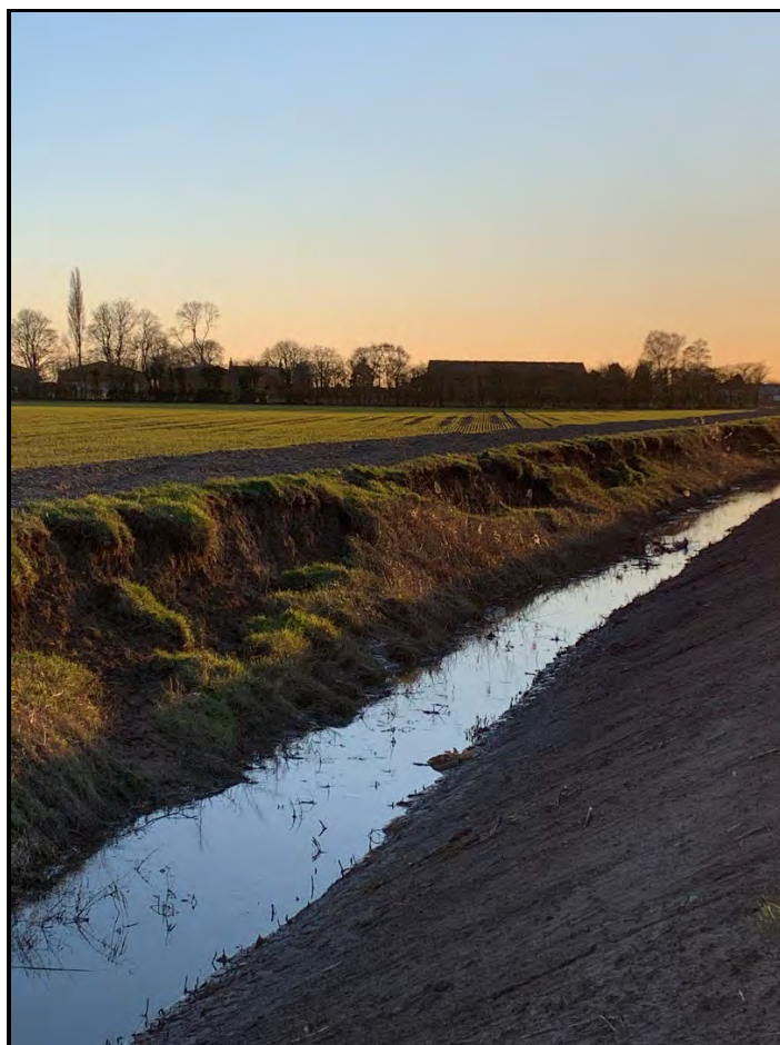
View of continuous length of slips in Moulton Mere post Storm Babet and Henk – January 2024
