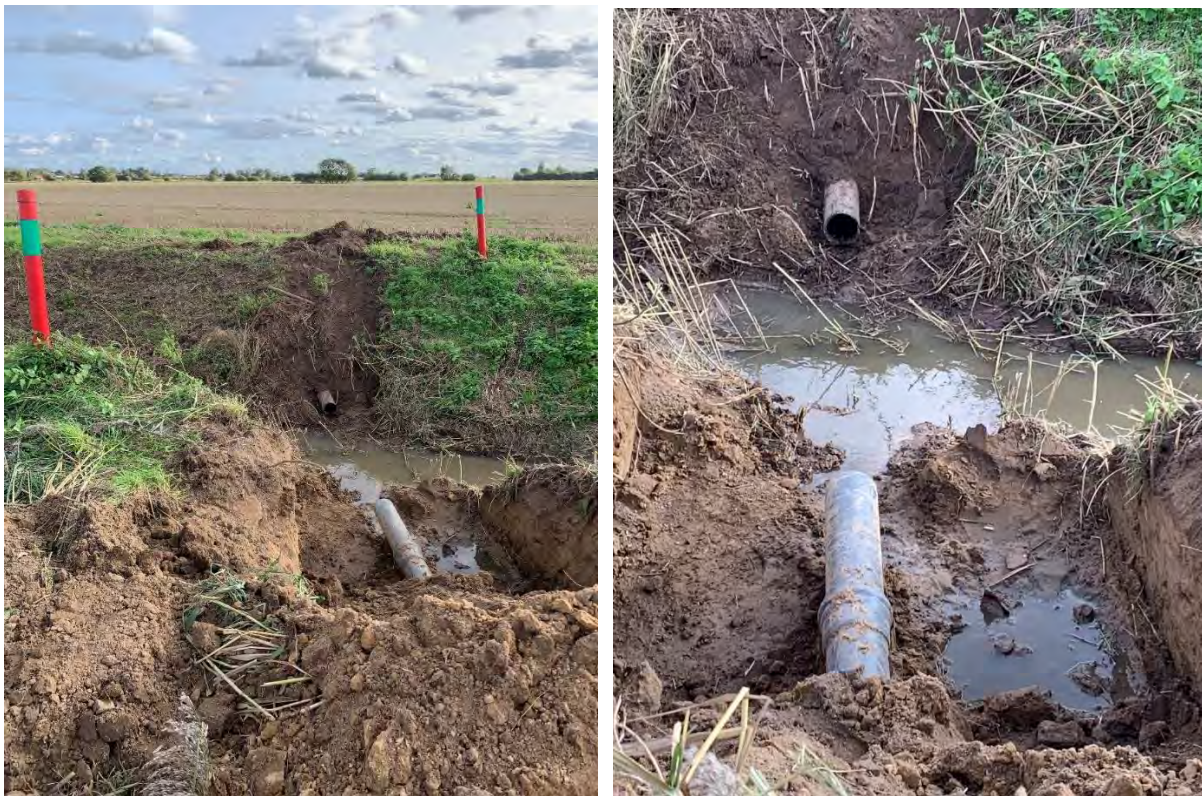
Views of the sewer having been cut back in readiness for repair. Note warning marker posts previously installed by the Board.
