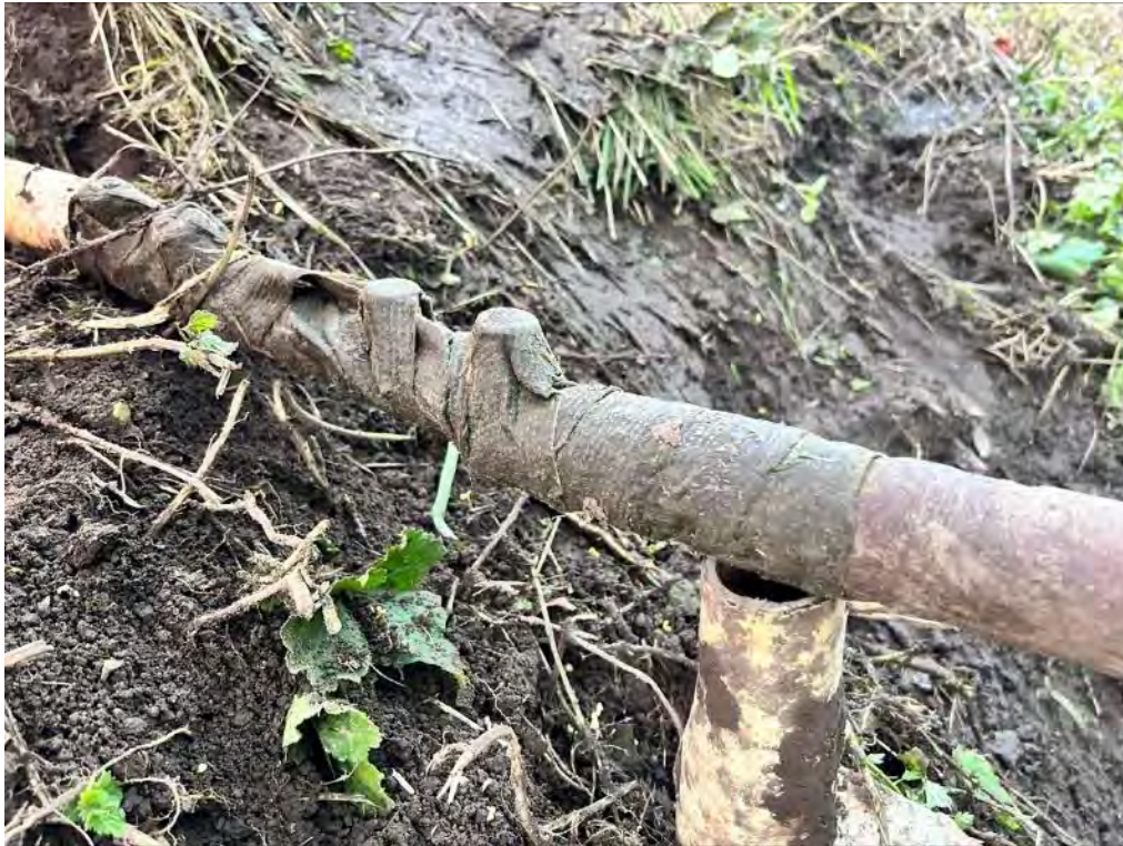
Another view of the repair – the prop under the duct can clearly be seen
