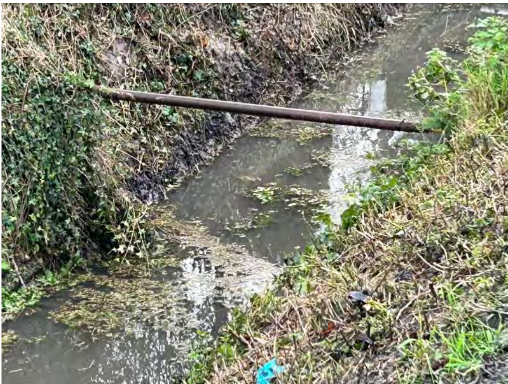
Photos showing the gas pipe in question within the steel duct following the damage. The damage was to the roadside end of the crossing, left above, and right below.
