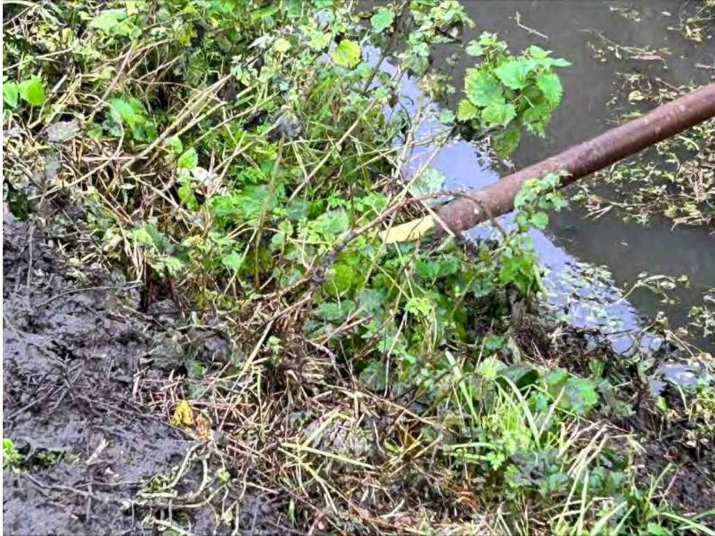
Close up of the damage showing part of the corroded steel duct missing and the yellow plastic pipe inside
