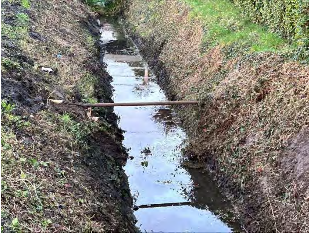
Another view of the repaired pipe. Repair is visible on the left
