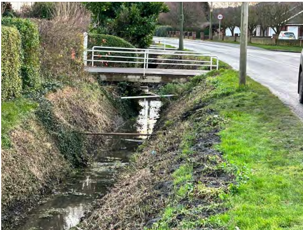
Photo showing the gas pipe (the one closest to the camera) following Cadent's repair
