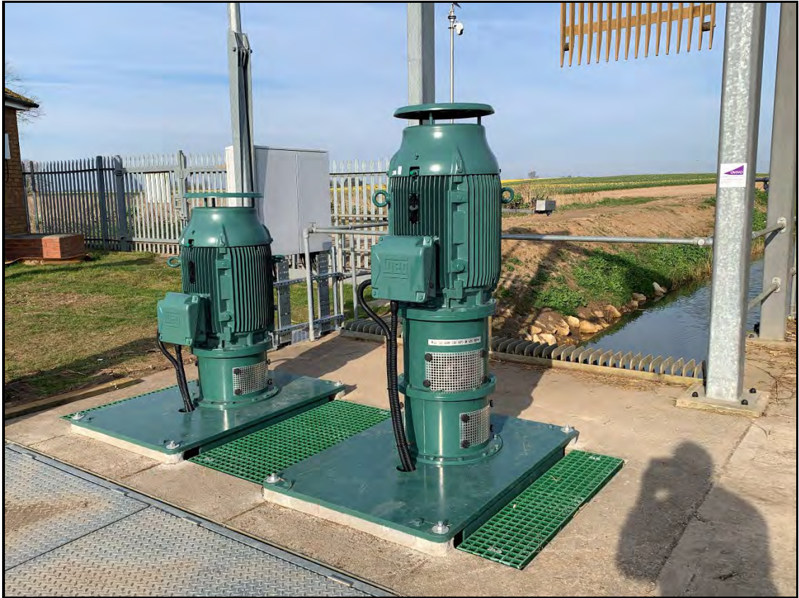
New pumps – view of motors. Right hand pump has backup PTO drive fitted
