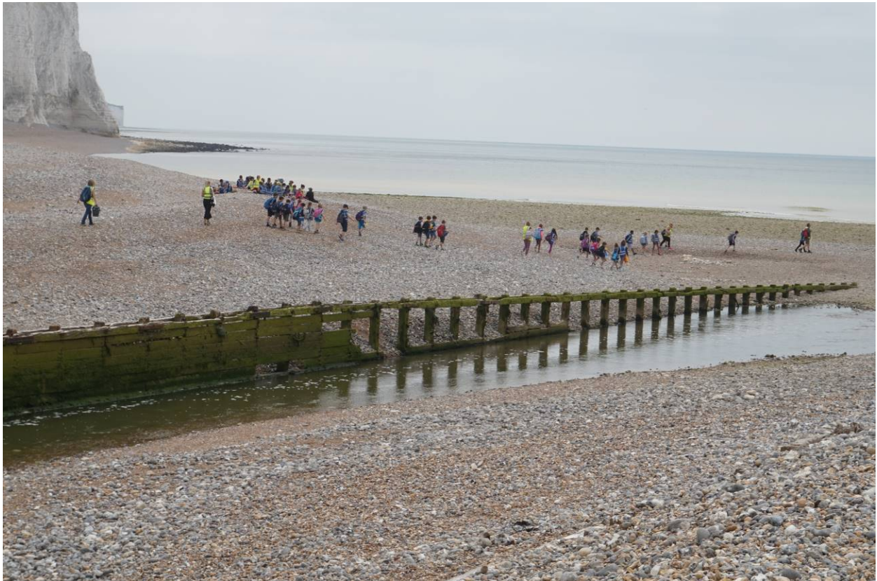
Existing retaining wall with loss of boards, no signage and safety issues
