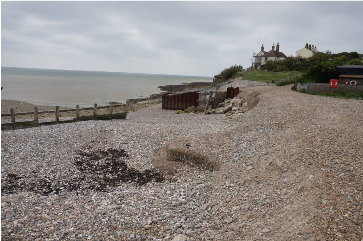
Failing training wall, where shingle could be placed
