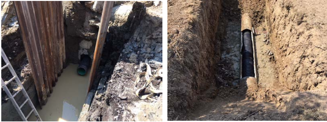
Photos showing the excavation required to get to the leak and damaged pipework
