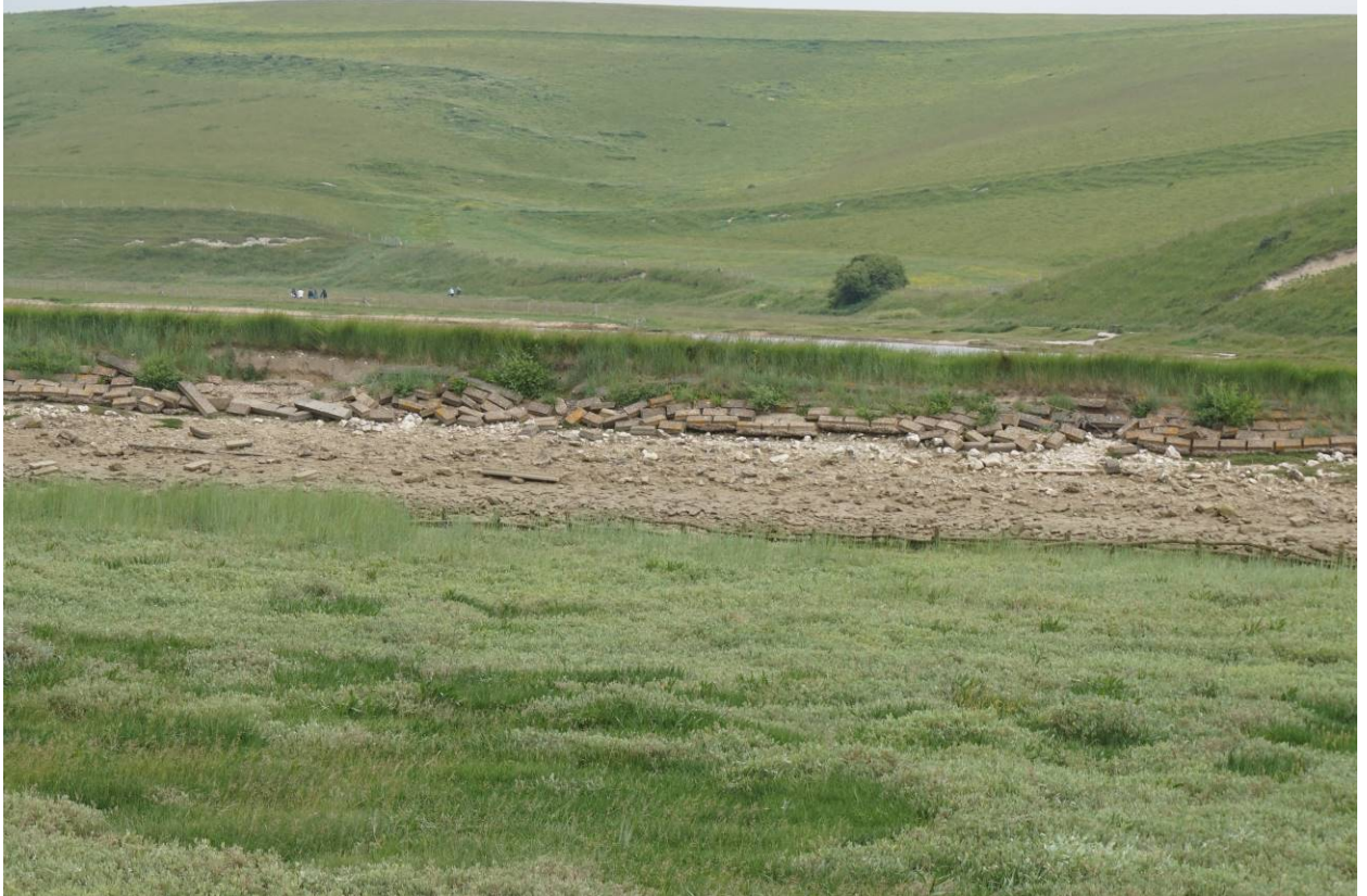
Revetment wall which has failed on the Eastern bank and which has part failed on the Western bank
