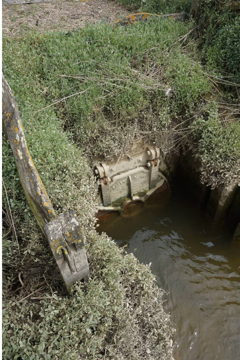
EA Flap Valve which is leaking water back into the IDD
