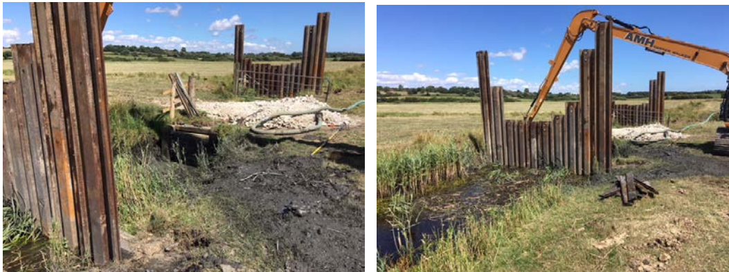
Cofferdams installed to isolate the structures and allow the boards to be removed and replaced in the dry
