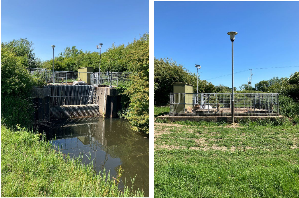
Figure 13: Existing Pumping Station at Drockmill
