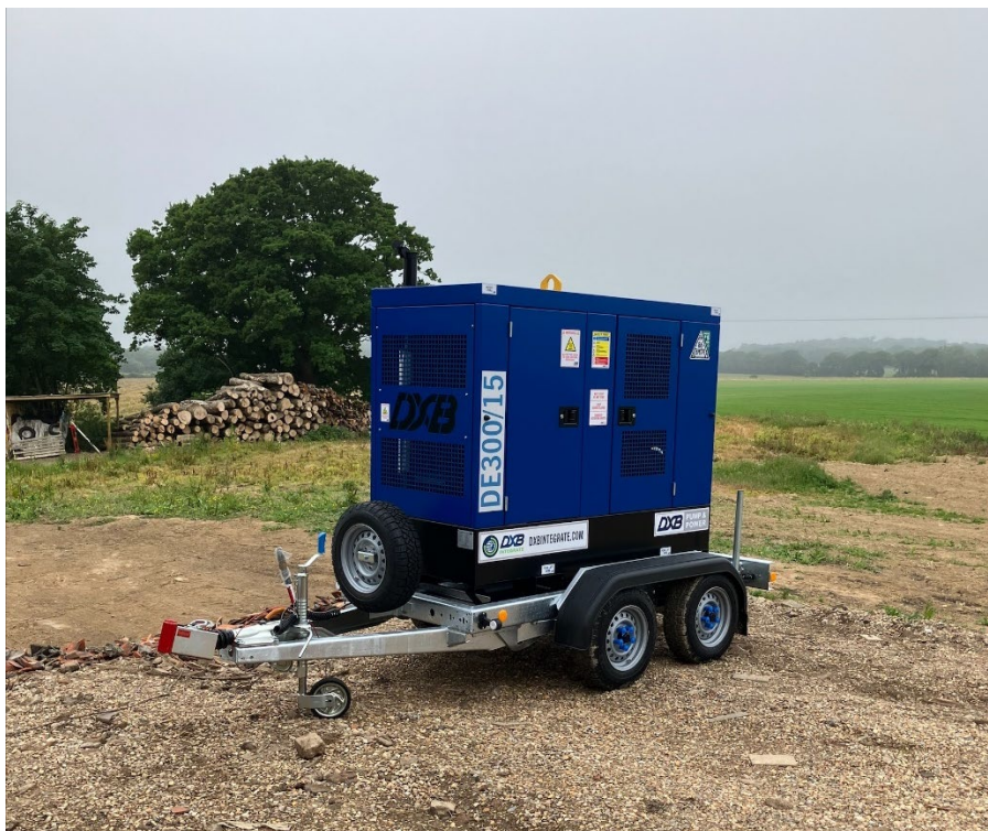
Figure 1: Mobile Pump in May 2025
