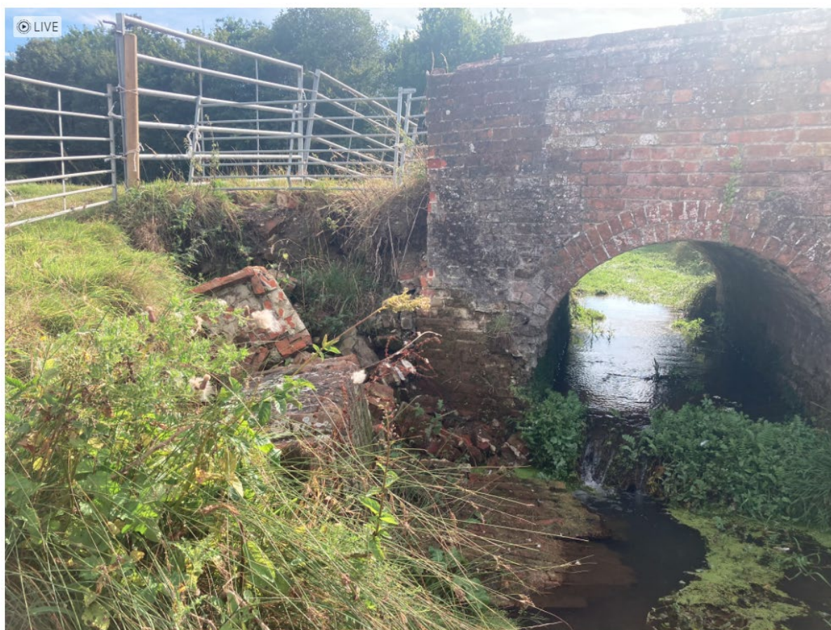
Photograph showing the damaged wingwall
