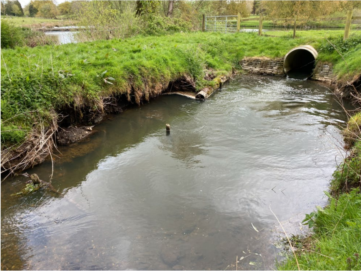
Bank erosion downstream of culvert
