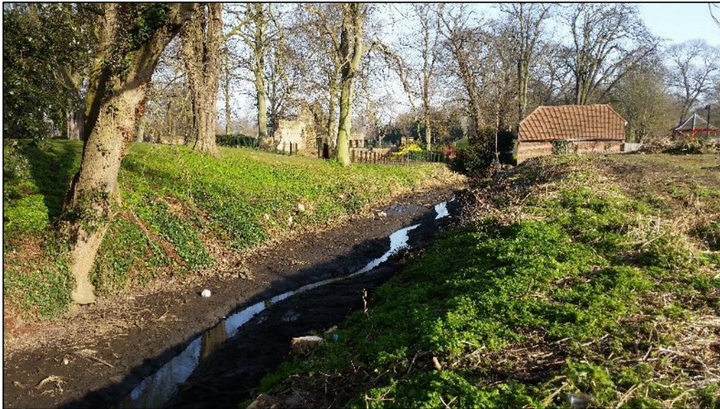
Photo 15 Seven Sisters drain project, before planting, but after excavation of new channel.
