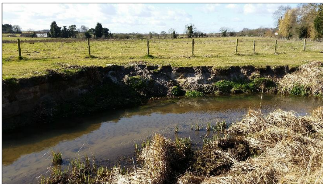
Photo 3 erosion from poaching on outside of meander bend. Lower bend shown in photo. Picture taken from right hand bank.
