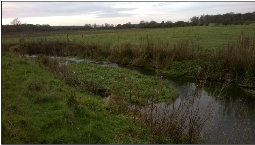
Photo 2 'Dig and dump' berm creation on near (left hand) bank. Now vegetated.
