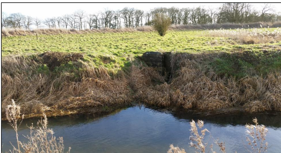
Photo 11 Showing concrete structures allowing water management of lake on right hand bank.
