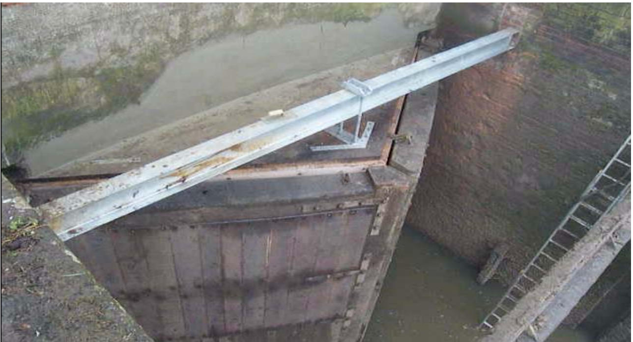
Refurbished gates and new canopy back in position alongside River Great Ouse
