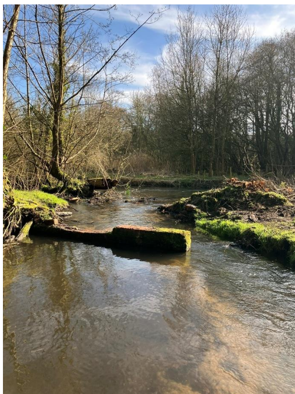
Before – Breached Culvert
