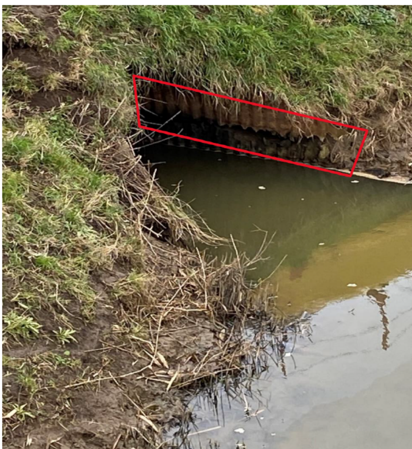
Picture showing erosion at the water line
