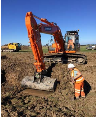
Dealing with a potentially significant archaeological find in area of new soke dyke excavation.
