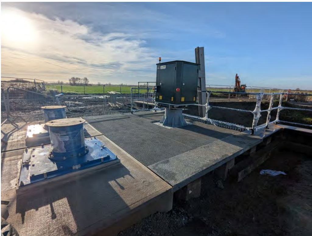
St Benets deck mounted weed cleaner system, wet well decking and fencing.
