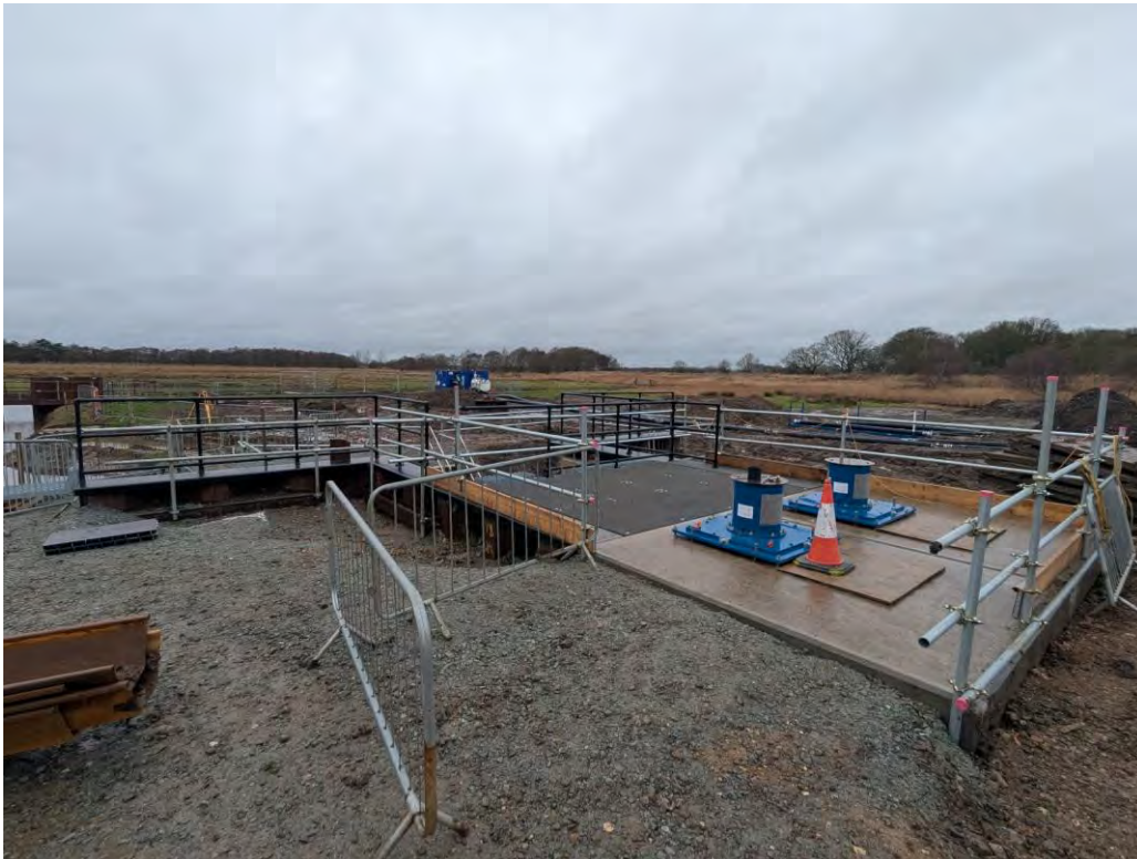
Horsey wet well decking, pump pedestals, pump support slabs and intake fencing
